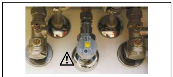
Fig.: Gas connection: Escaping gas may cause poisoning or the risk of explosion
